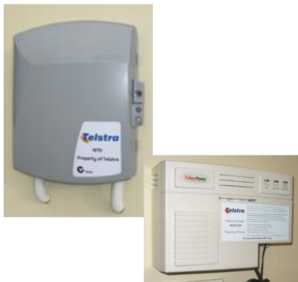
Outdoor Termination Device & Power Supply
